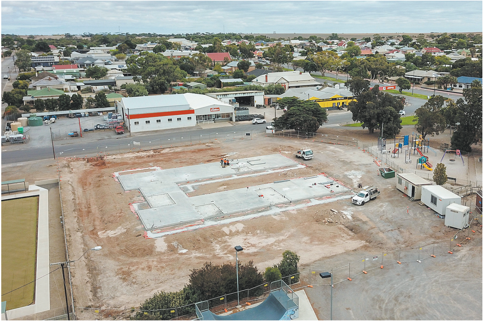
FROM THE GROUND UP... The current state of the Southern Yorke Peninsula Childcare Centre construction work at Minlaton.
